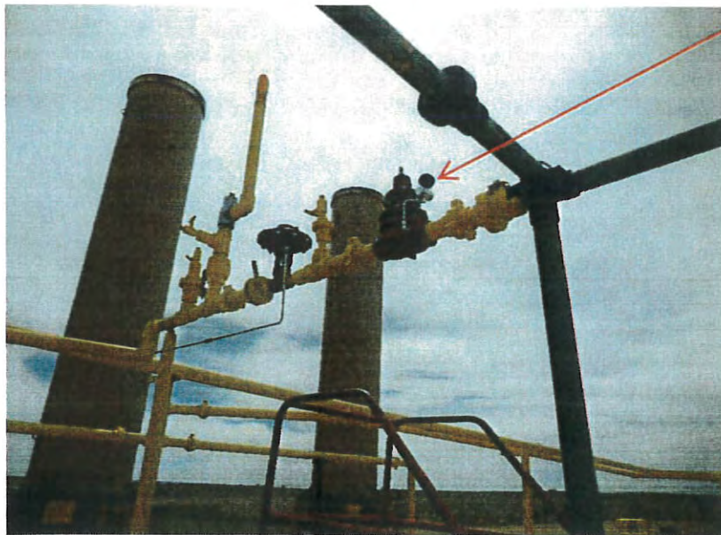
LP header w/ second back pressure regulator
