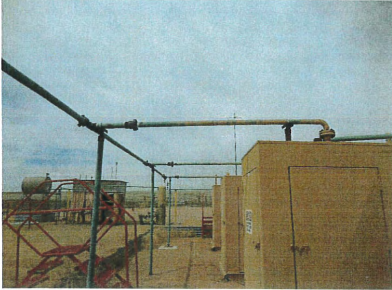
Common LP header tie in
